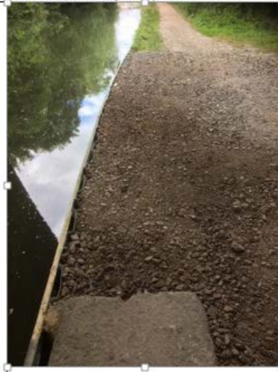
GU-178-007 – Railway Bridge Towpath Wall recently reconstructed. Grass verge to be reinstated
